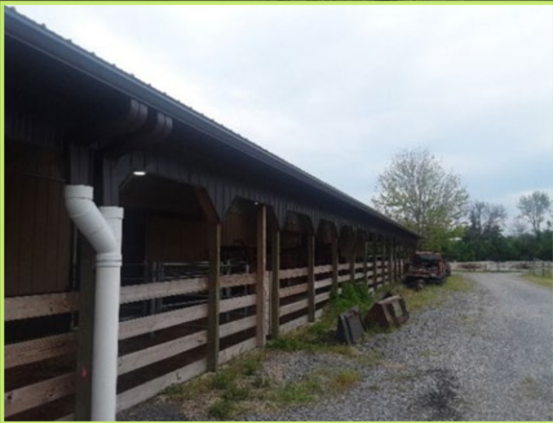
1 - Roof Water Collection System
